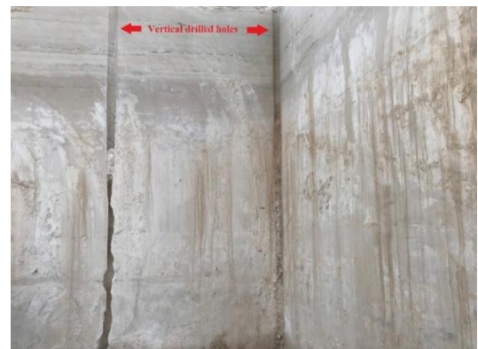
Fig. 4. An example of remaining traces of vertical drilled holes after the block cutting.
