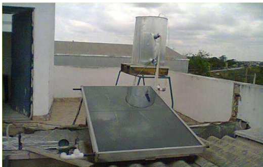
Figure 2. Solar Heating System Installed for Configuration II: (Glass)
