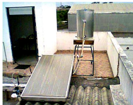
Figure 1. Solar Heating System Installed for Configuration I: (Polycarbonate)
