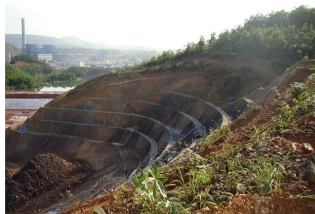
Fig. 8 The Storm Water Drainage and Benching along the Hilly Slopes of Ash Pond.
