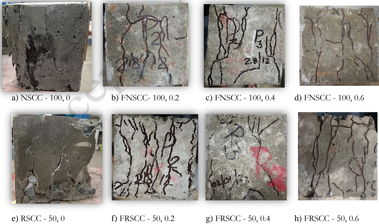
Fig. 9. Crack propagation in NAC and RAC without and with use of PP Fiber.
