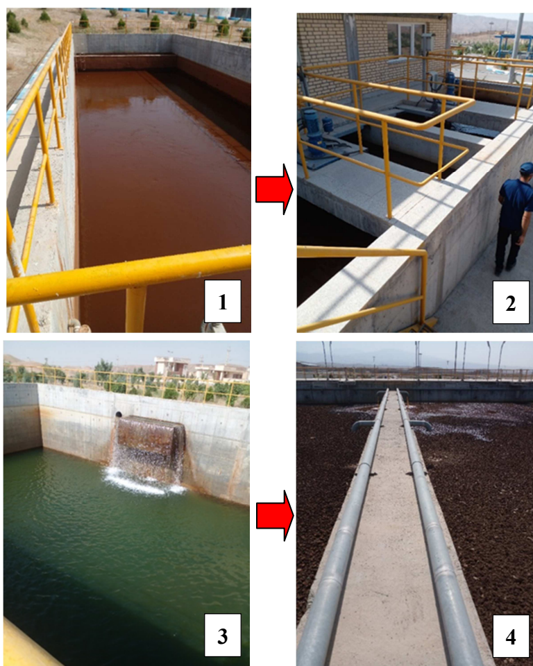
Figure 8. Stages of wastewater treatment of the seventh drinking water treatment plant in Tehran
