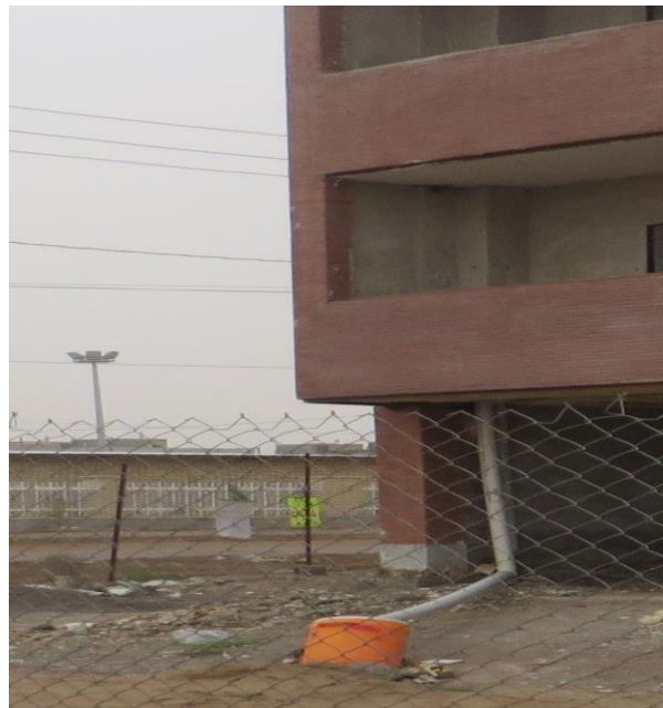
Fig. 1. A view of collecting rainwater by PVC pipes
