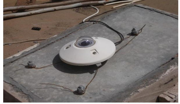
Figure 8: Pyranometer installed in CNES on a tilt angle of 15°.
