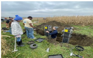
Controlled Drainage (South Dakota site)
